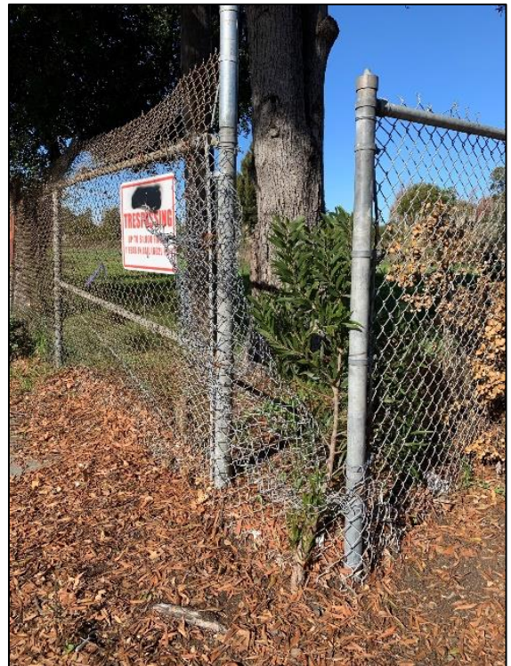
Figure 12. Cut fence corner at the end of Wood Street.
