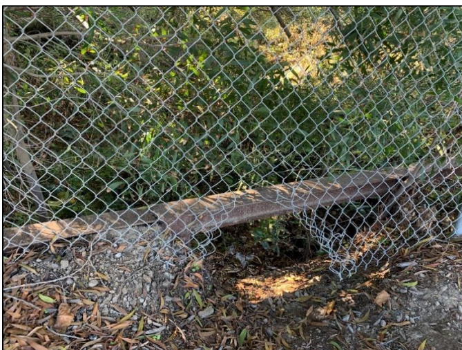
Figure 7. Hole cut into fence.
